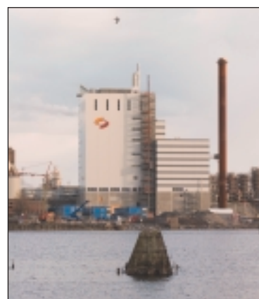
The CTMP construction plant at Stora Enso Skogshall's mill.
